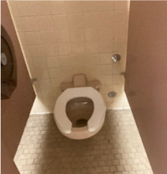
Fig p-20 - Water Closet
