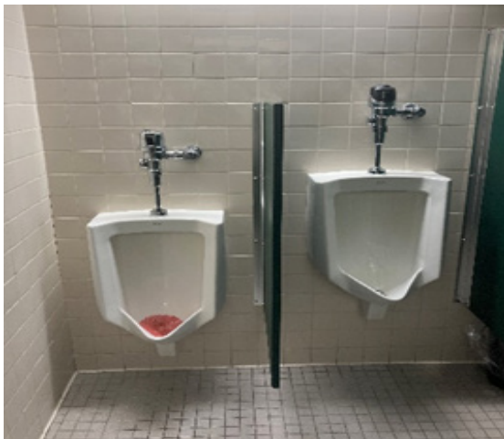
Fig P-9 - Urinals at ADA Restroom
