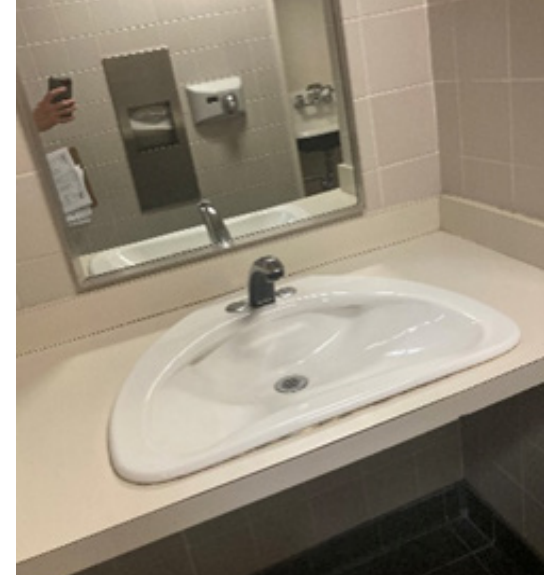
Fig p-23 - Lavatory at ADA Restroom
