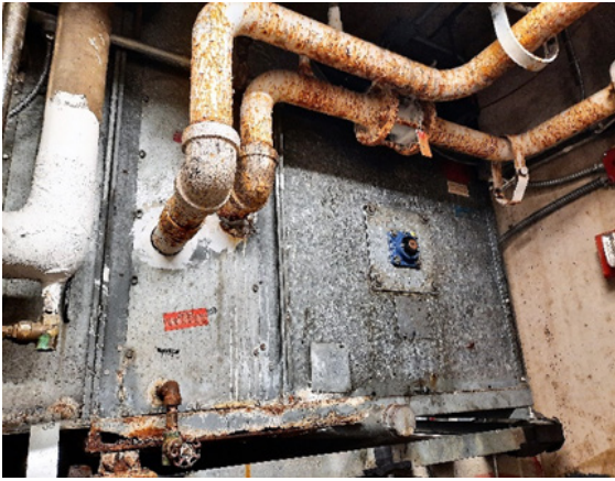
Fig H-13 - Air Handling Unit Corrosion
