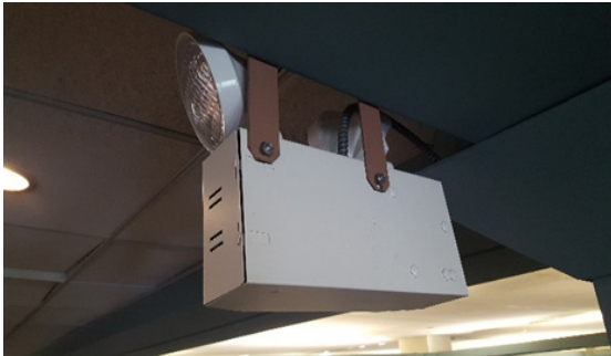
Fig E-8 - Unitek Battery Light Mounted Below ADA Height
