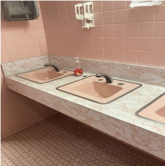
P-12 - Lavatories at Women's Restroom
