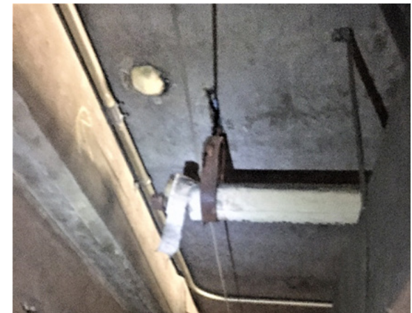
Fig H-12 - Abandoned Piping Risers
