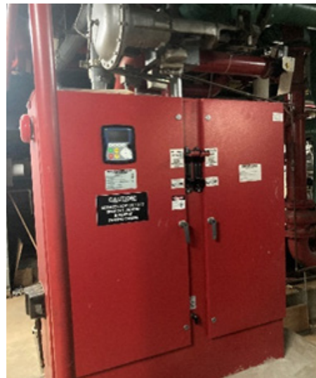
Fig P-33 - Fire Pump Controller
