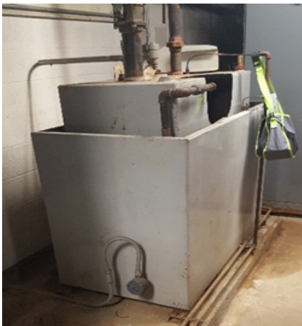
Fig E-12 - Generator Fuel Tank Cut Open and Drained
