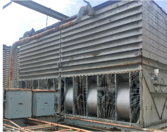
Fig H-8 - Abandoned Cooling Tower
