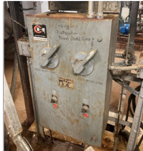
Fig P-29 Sump Pump Control Panel
