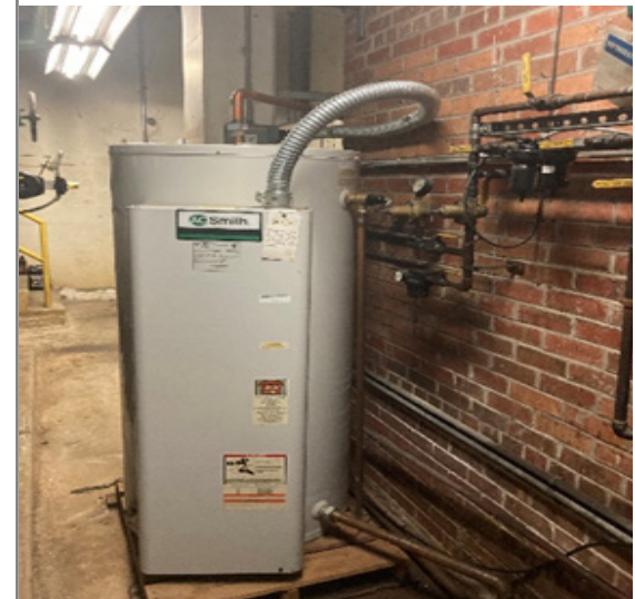
Fig P-3 Electric Water Heater
