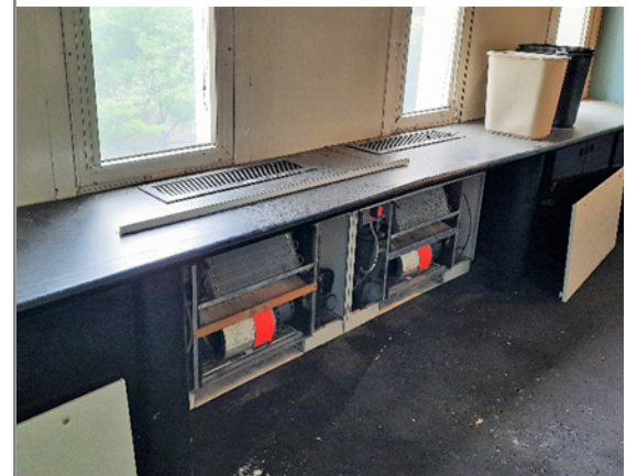
Fig. H-2 - Typical Fan Coil Units
