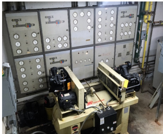
Fig. H-11 - Existing Control Panels
