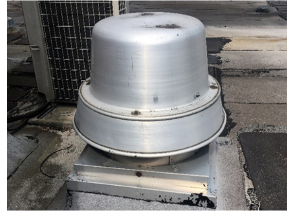
Fig H-9 - Typical Toilet Exhaust Fans
