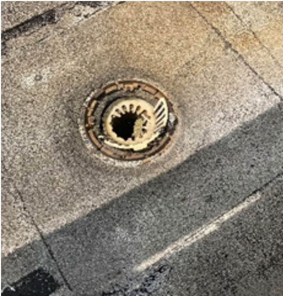
Fig P-27 - Roof Drain
