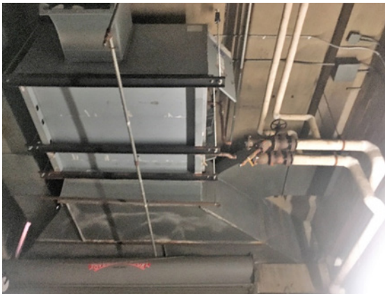
Fig H-4 - Garage Heating & Ventilating Unit
