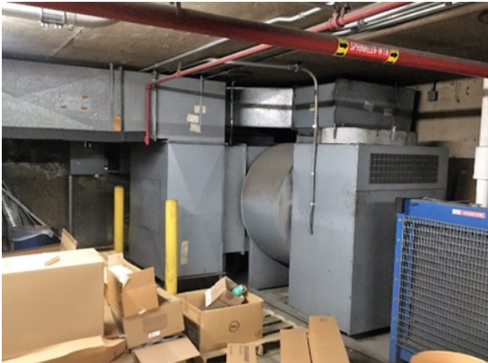
Fig H-3- Garage Exhaust Fans
