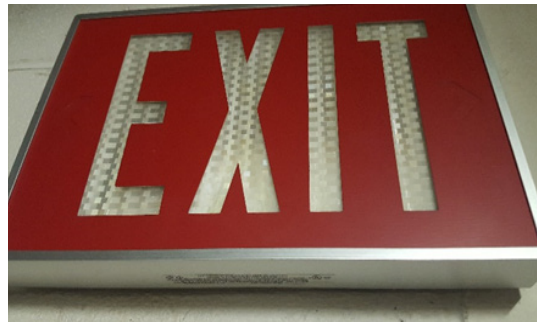
Fig E-9 - Exit Sign Illuminated with Radioactive Gas
