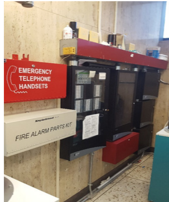
Fig E-14 - Fire Alarm System Control Panel
