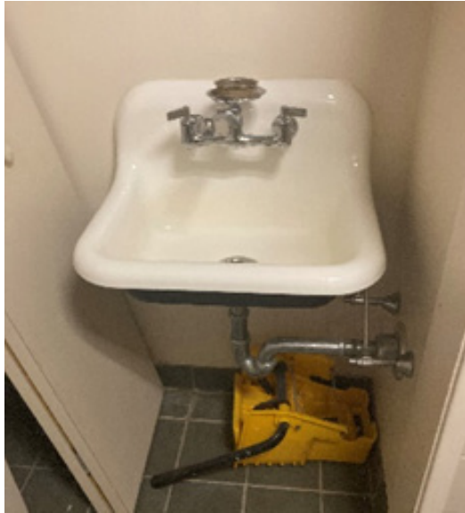
Fig P-22- Utility Sink at ADA Restroom
