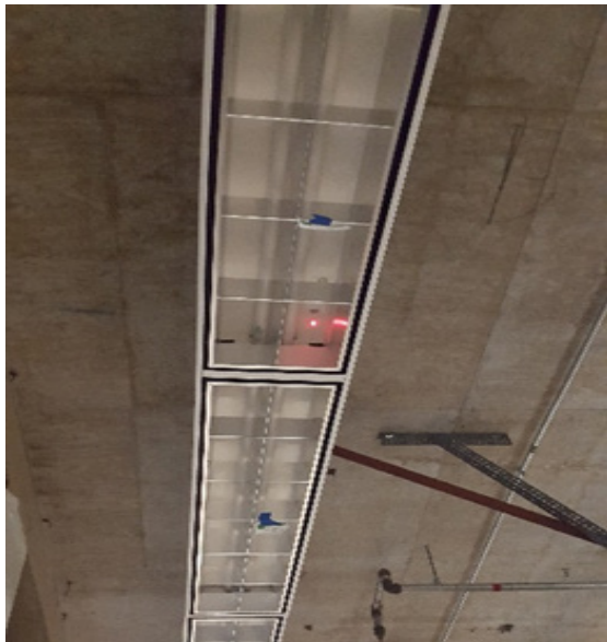
Fig E-7 - Emergency Battery in Light Fixture Indicated by Red Light
