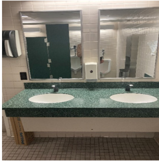
Fig P-7 - Lavatories at ADA Restroom
