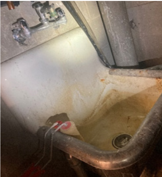
Fig P-21 - Utility Sink at Janitor's Room
