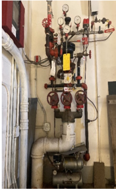
Fig P-36 - Preaction Valve and Standpipe Manifold
