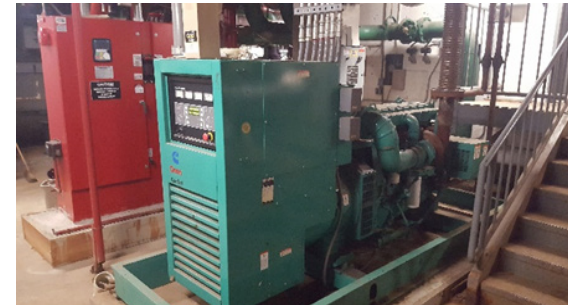
Fig E-11 - Emergency Generator
