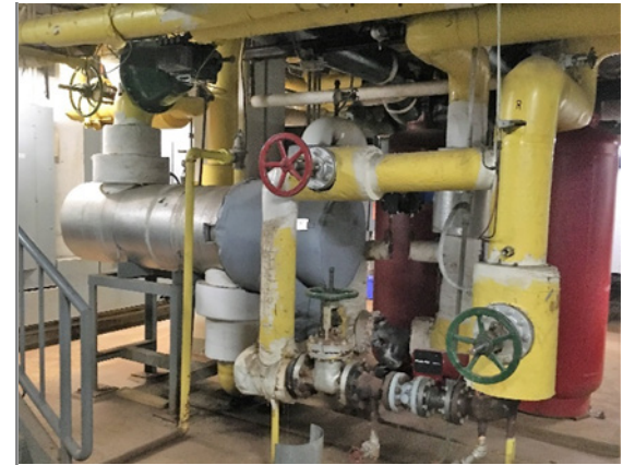
Fig H-5 - Hot Water Heat Exchanger
