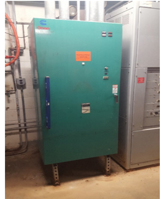
Fig E-13 - Emergency, Automatic Transfer Switch
