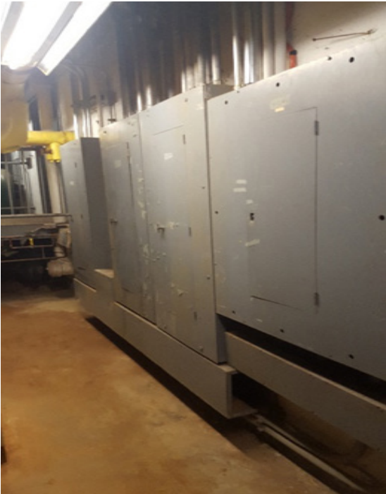
Fig E-3 - Original Boiler Room Panels
