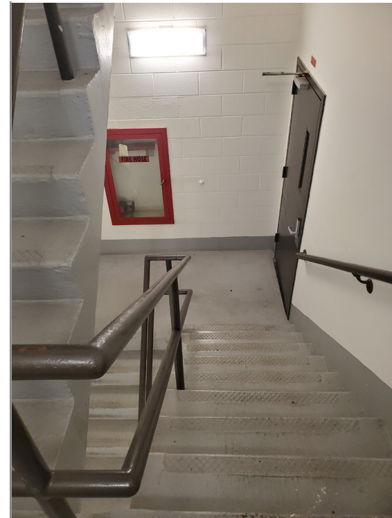
Typical egress stair with standpipe. The existing vertical enclosure meets the 2 hr fire rating requirement. Handrails and guardrails need to be upgraded to meet current codes.
