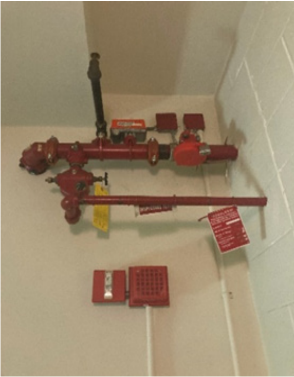
Fig P-35 - Wet Floor Control Valve
