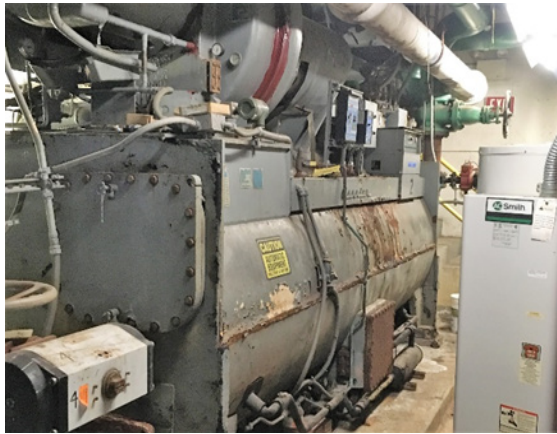
Fig H-7 - Abandoned Chillers
