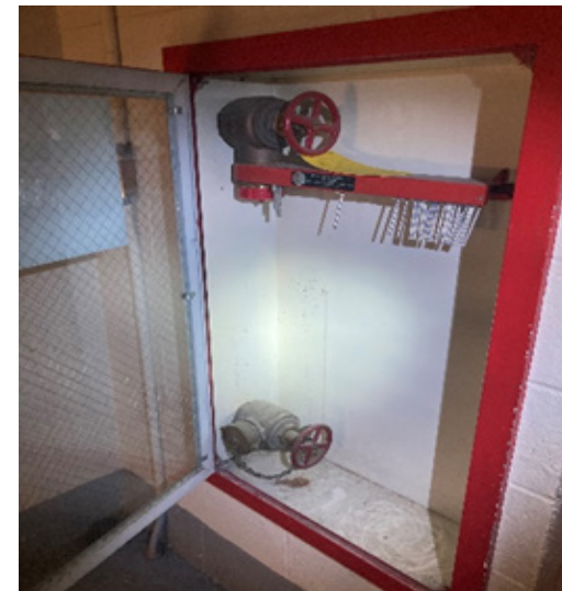
Fig P-34 - Fire Department Hose Connections
