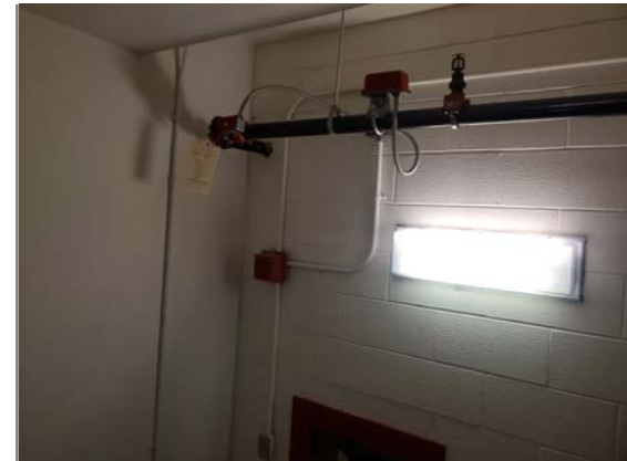
The existing fire sprinkler system and other fire protection systems will need to be reconfigured and upgraded to accommodate the building uses and to meet current code requirements.
