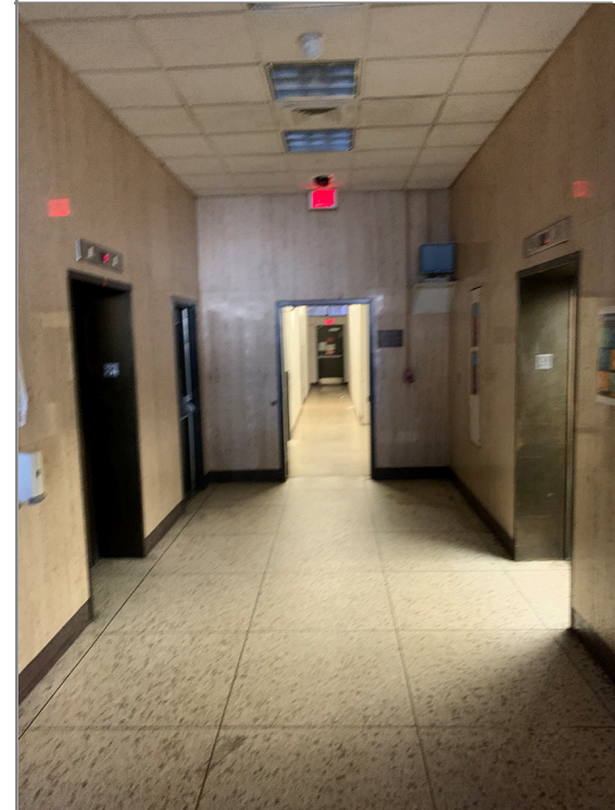
First floor elevator lobby. In general, the elevator lobby on each floor will need to be enclosed with fire rated assemblies.
