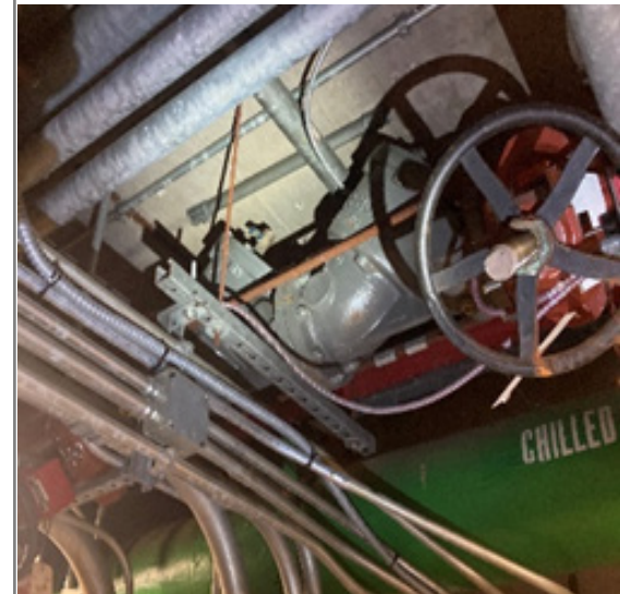
Fig P-30 - Fire Protection Backflow Preventer
