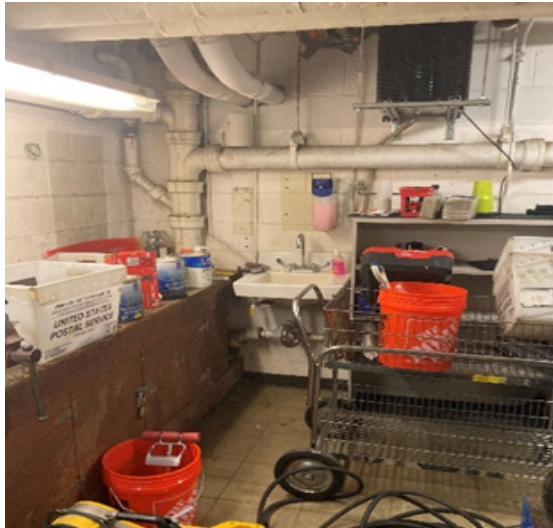
Fig P-4 - Sanitary Stack in Basement
