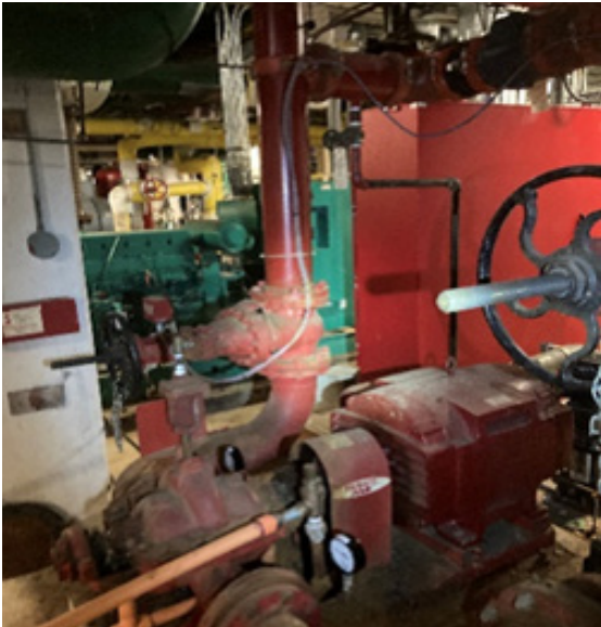
Fig P-31 - Fire Pump
